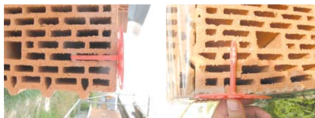
Fig. 3 Inappropriate anchorage of adhesive anchor is demonstrated on the left side and appropriate application is shown on the right side
