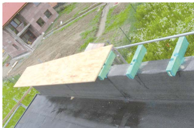
Fig. 2 Part of the flat roof (to create space for the insulation of attic)
