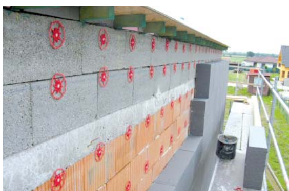
Fig. 4 Application of special thermal baseboard of thermal insulating system and arrangement of adhesive anchors on the wall with application of thermal insulating system
